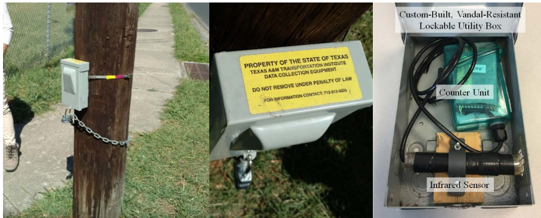
Figure 10. TRAFx Trail Counter Deployed and the Inside of the A/C Disconnect Box.
